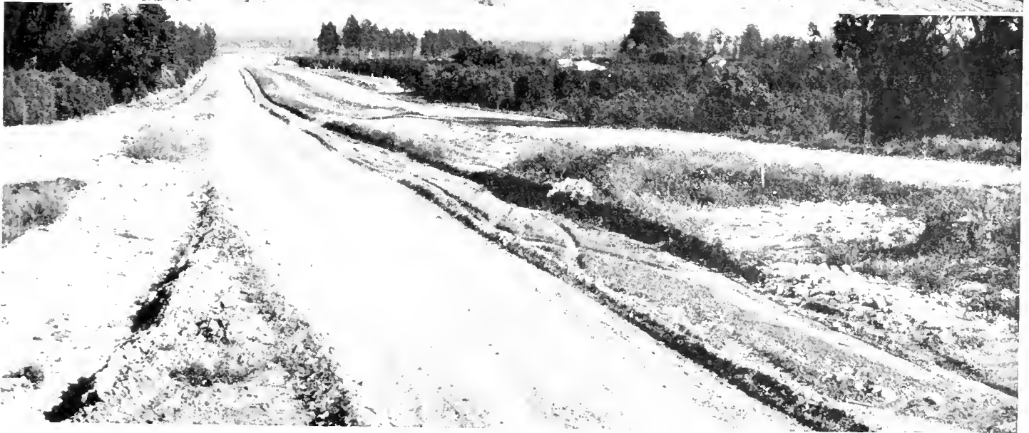
UPPER—Looking northerly along construction toward end of job at First Street Overcrossing. CENTER—Looking southerly along construction from top of fill for Newport Avenue Undercrossing. LOWER—Looking southerly on construction from fill for Route 2.43 separation at Tustin Avenue.
